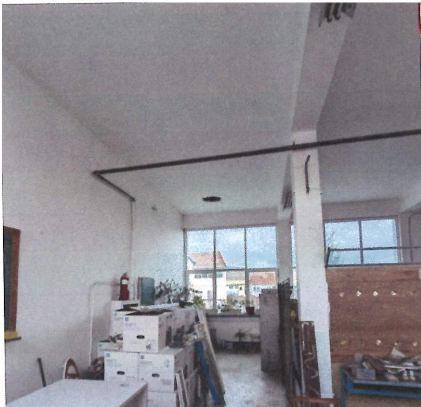
Photo 6 – Photo of the Electric Workshop block. One can see the structure in frames and in the left side the reinforced concrete walls
