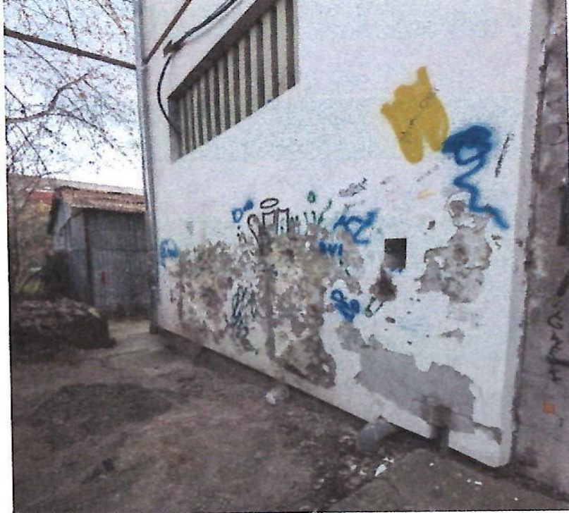
Photo 11 – Photo of the posterior entrance on the transformer station. One can see that the thermal insulation has been vandalized.
