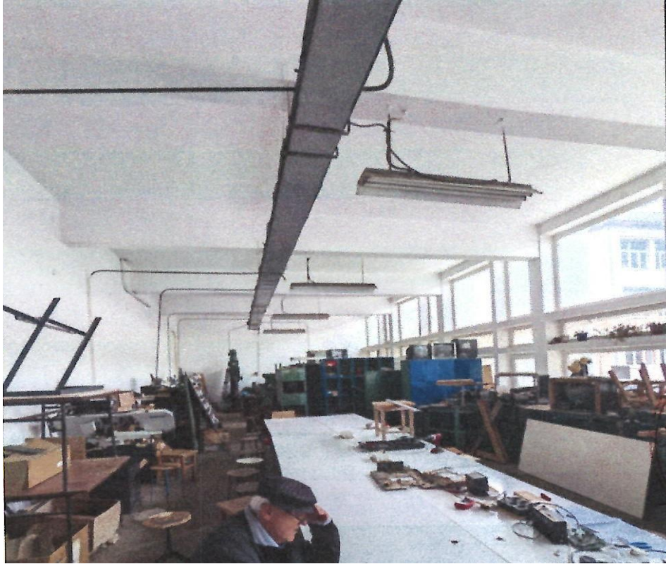
Photo 7 – Photo of the Gf+2F block, at Gf the Electrical mechanics workshop. One can see the median wall of masonry and the reinforced concrete frames
