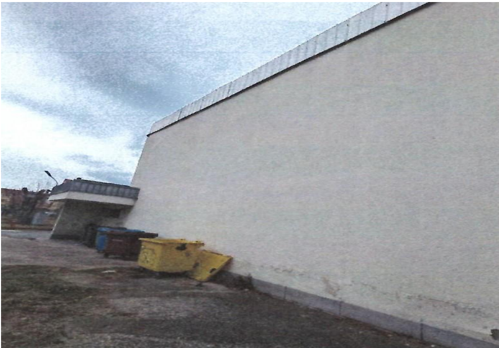
Photo 8 – Transversal right wall. One can see a wetting of the wall in the lower side, most probably due to the pavement with reverse slope.
