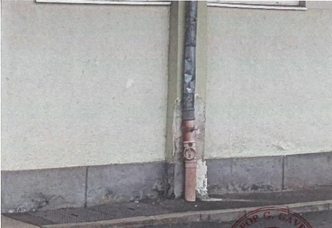
Photo 3 – Main entrance – damaged pipe
