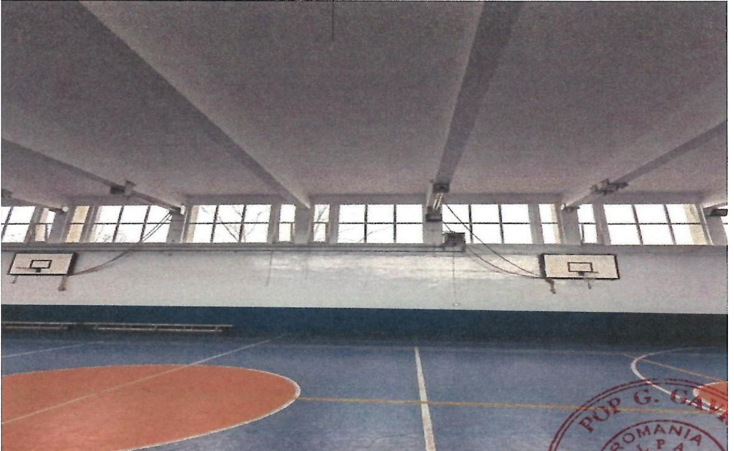
Photo 5 – Viewing from inside the gym hall, one can detect the main beams, the pillars and the longitudinal wall from N limit
