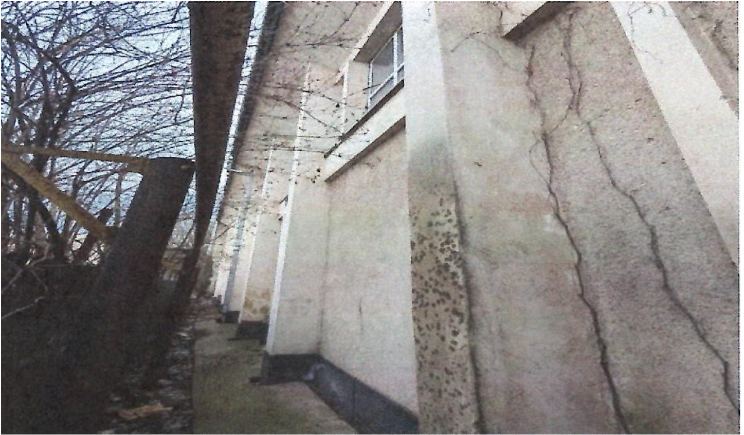
Photo 7 – Longitudinal wall with its entrance from the north side. One can see that the pavement detached itself from the construction and does not provide the removal of rainwater from the building.
