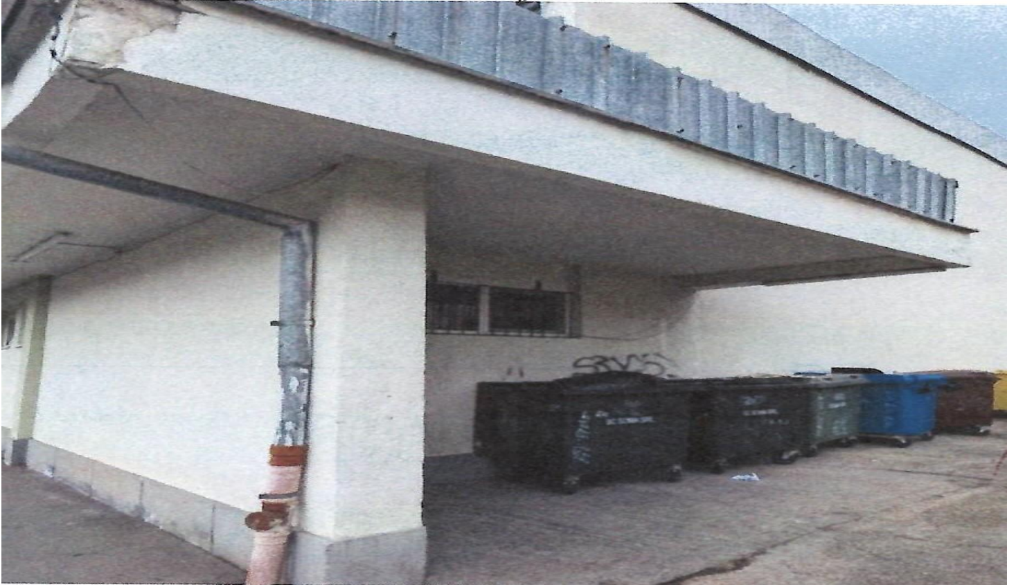
Photo 9 – Degradations of the concrete terrace plaster over the terrace.
