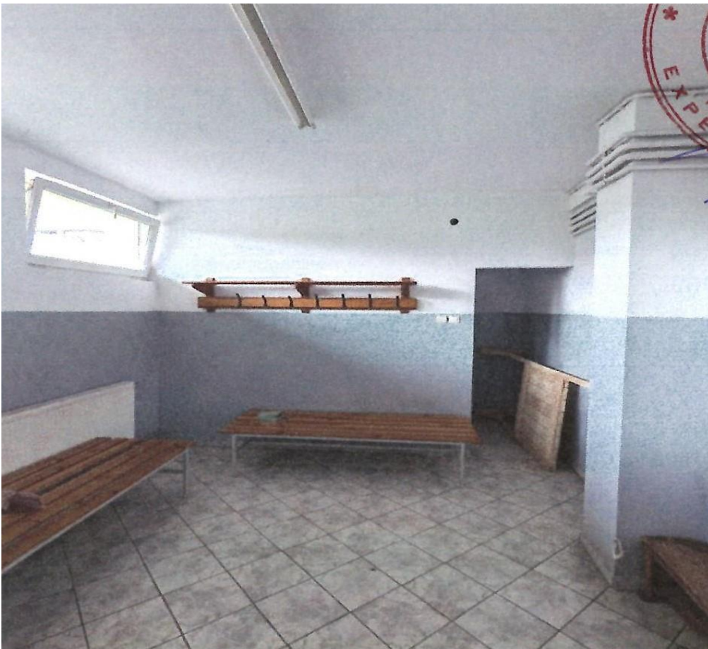
Photo 4 – Locker rooms – in the right side one can see a main pillar
