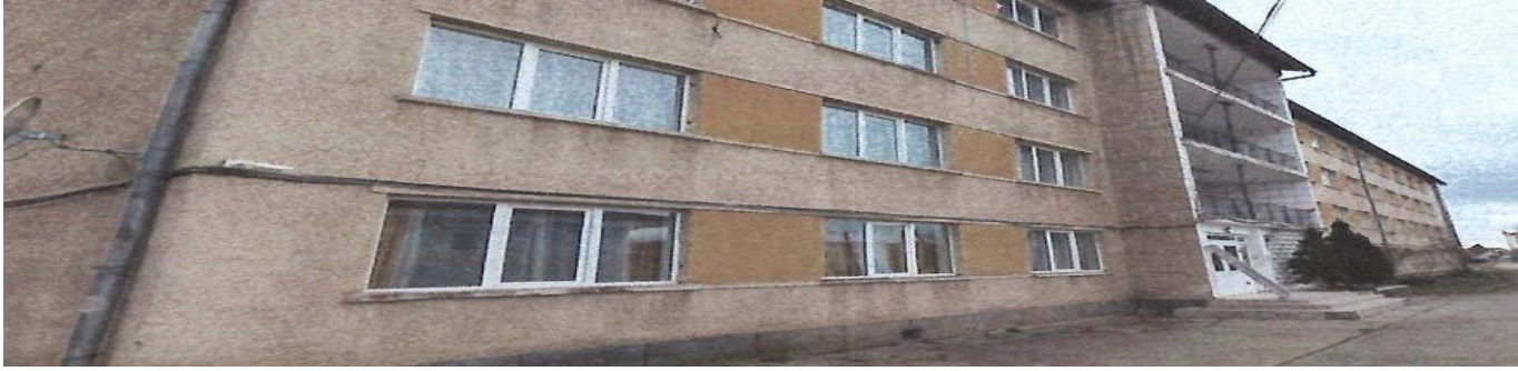
Photo 1 – Main entrance. Some infiltrations can be seen at the Annex socket.
