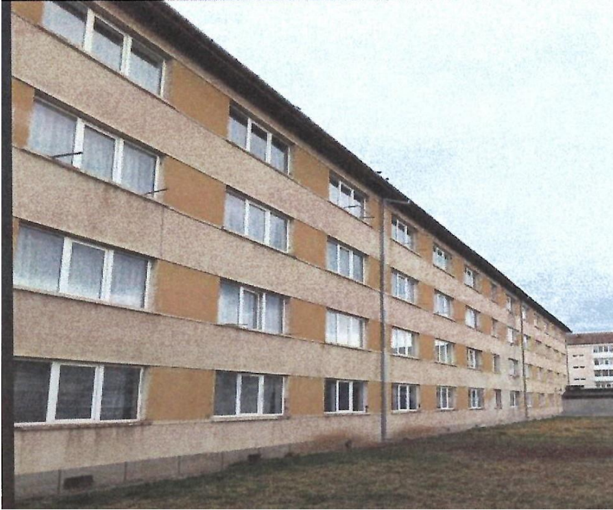
Photo 3 – Main entrance; damaged pipehole
