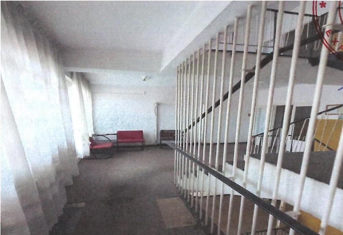
Photo 6 – Staircase area; one can see the reinforced concrete frames that support also the flight of stairs
