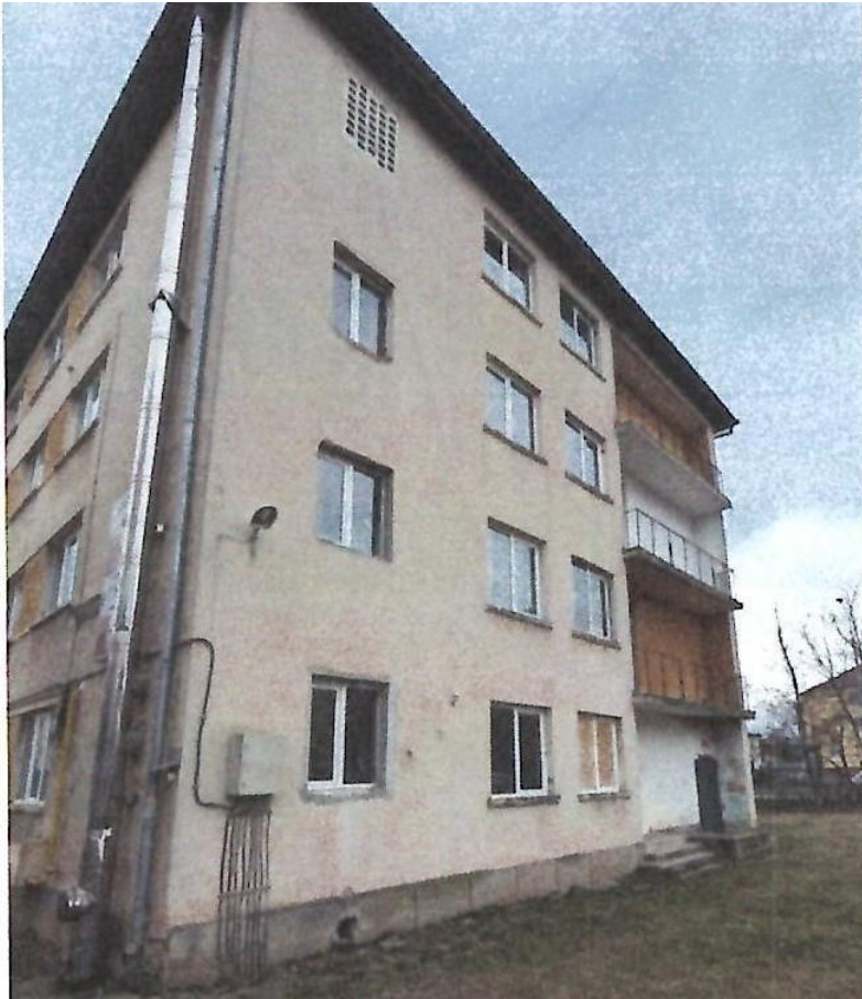
Photo 2 – Entrance from Vasile Aaron street, one can see the absence of a perimetral pavement
