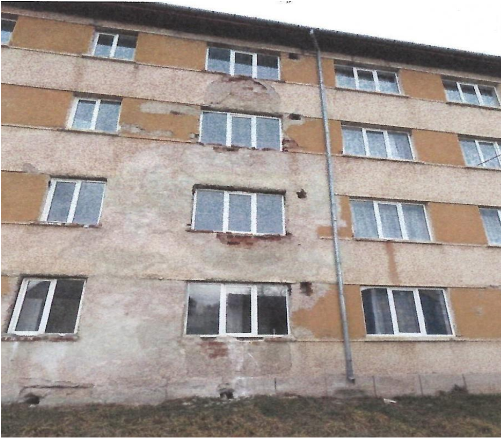
Photo 9 – Entrance from Electricienilor street. One can see the absence of the pavement and parts with the plaster fallen
