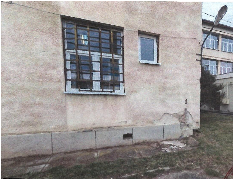
Photo 6 - entrance photo. one can see some parts on which the plaster fell and the absence of the guardrail on one side
