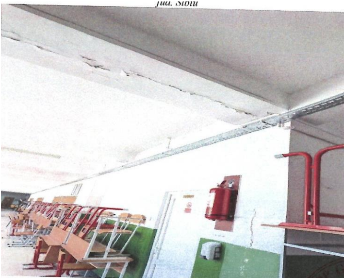
Photo 10 - Joint between section A and C improperly treated
