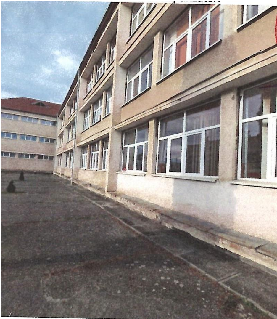
Photo 11 – Entrance from Electricienilor street. One can see the brice-soleil with the plaster fallen.
