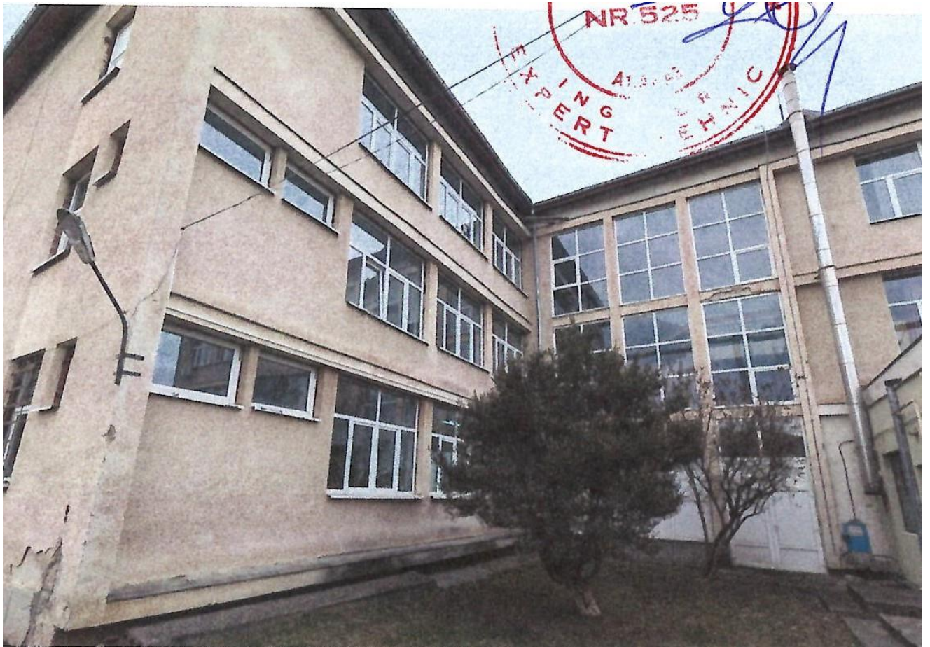
Photo 3 – Photo from thermal system. Some plaster degradations can be seen.
