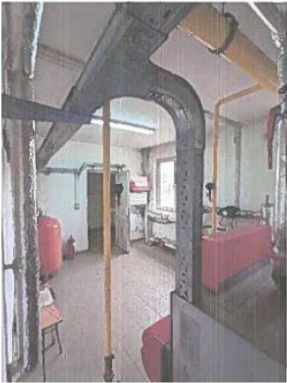
Photo 5 – Heating system room
