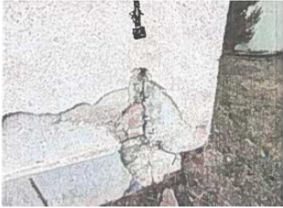
Photo 10 - Exterior plaster and base degradations
